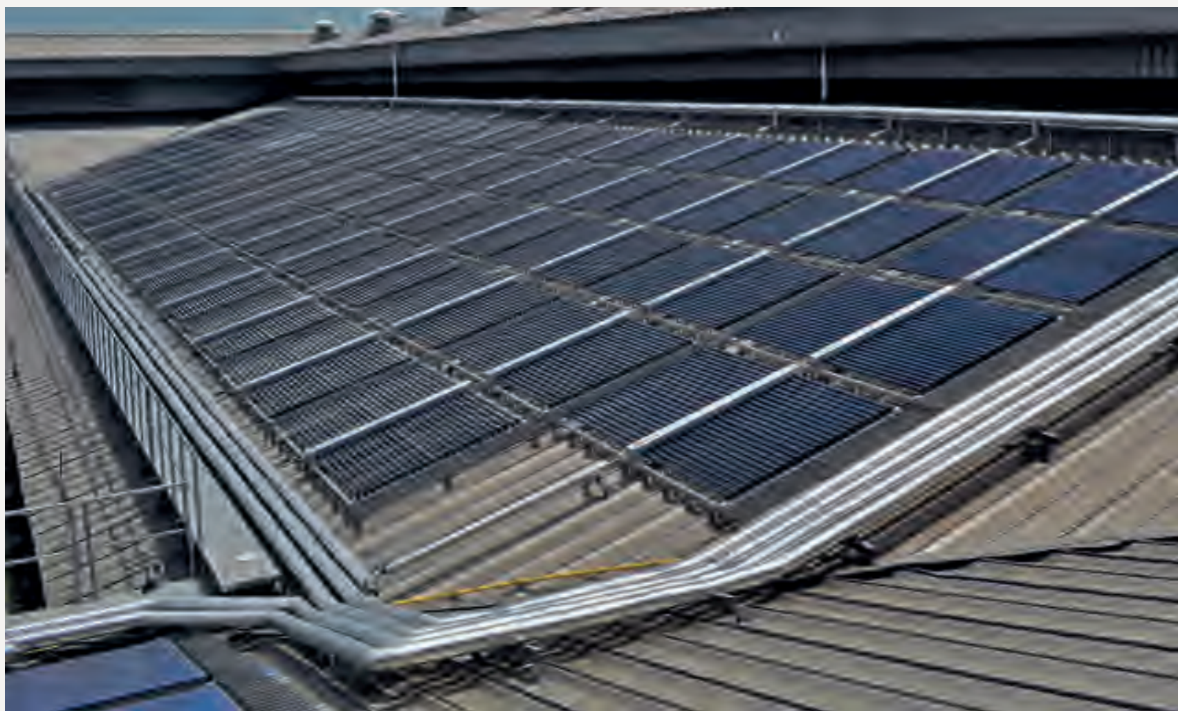
Solar panels cover the roof of ECCO's tannery in Thailand.
