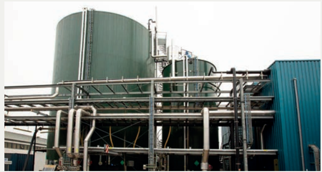
The waste water treatment plant in Dongen, the Netherlands.
