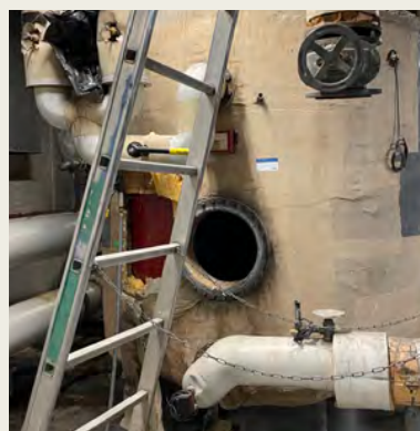
Removal of outdated central boilers at Bella Center has in 2022 contributed to energy optimization.
