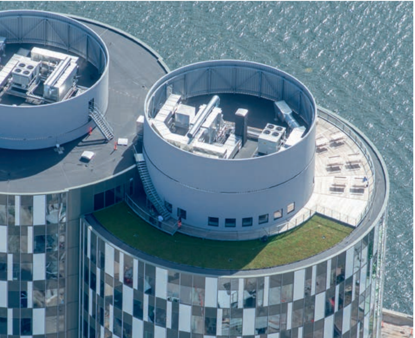
The roof tops of Portland Towers in Copenhagen are protected by Nordic Waterproofing's products, bitumen roof felt and green roof.
