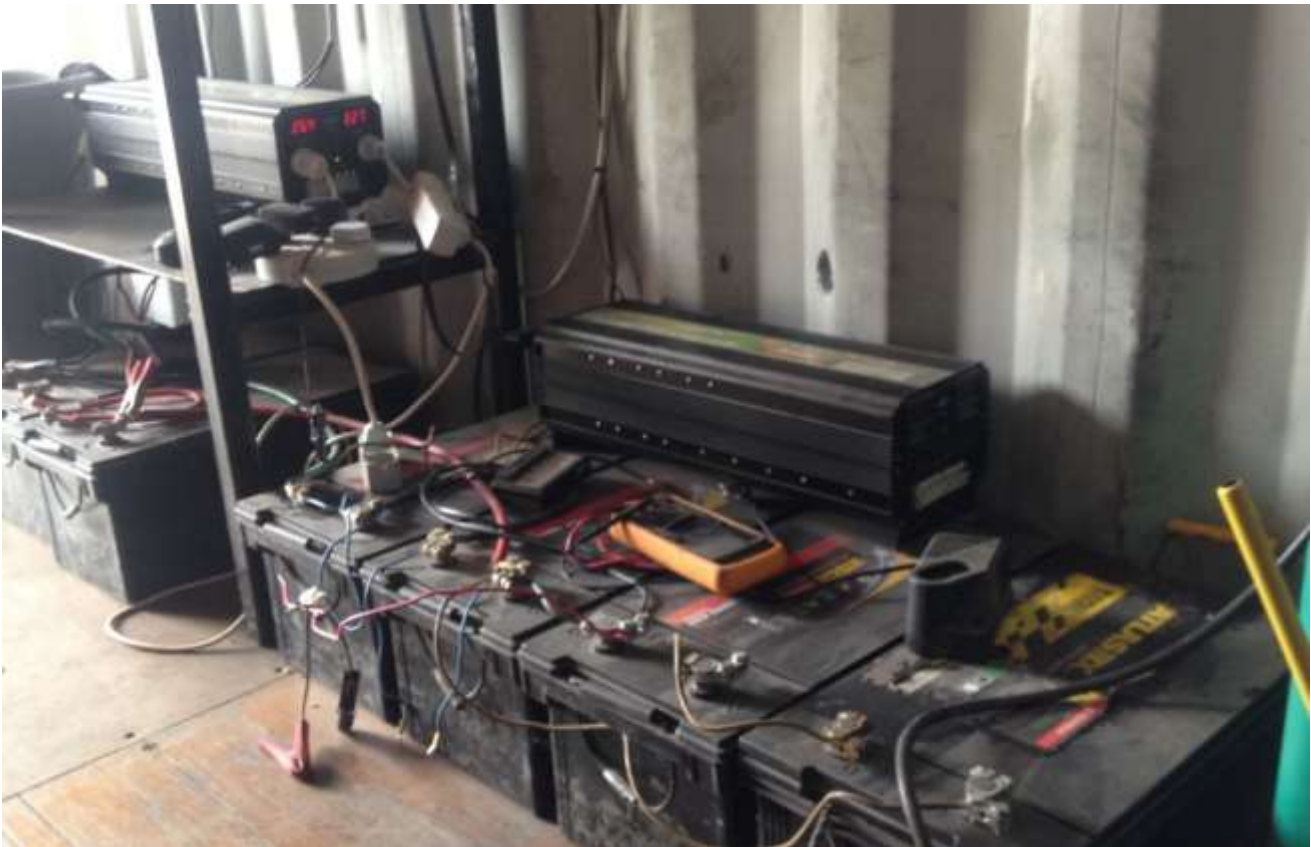
4 solar panel installations with in all 2 x 5000 Watt inverters.
