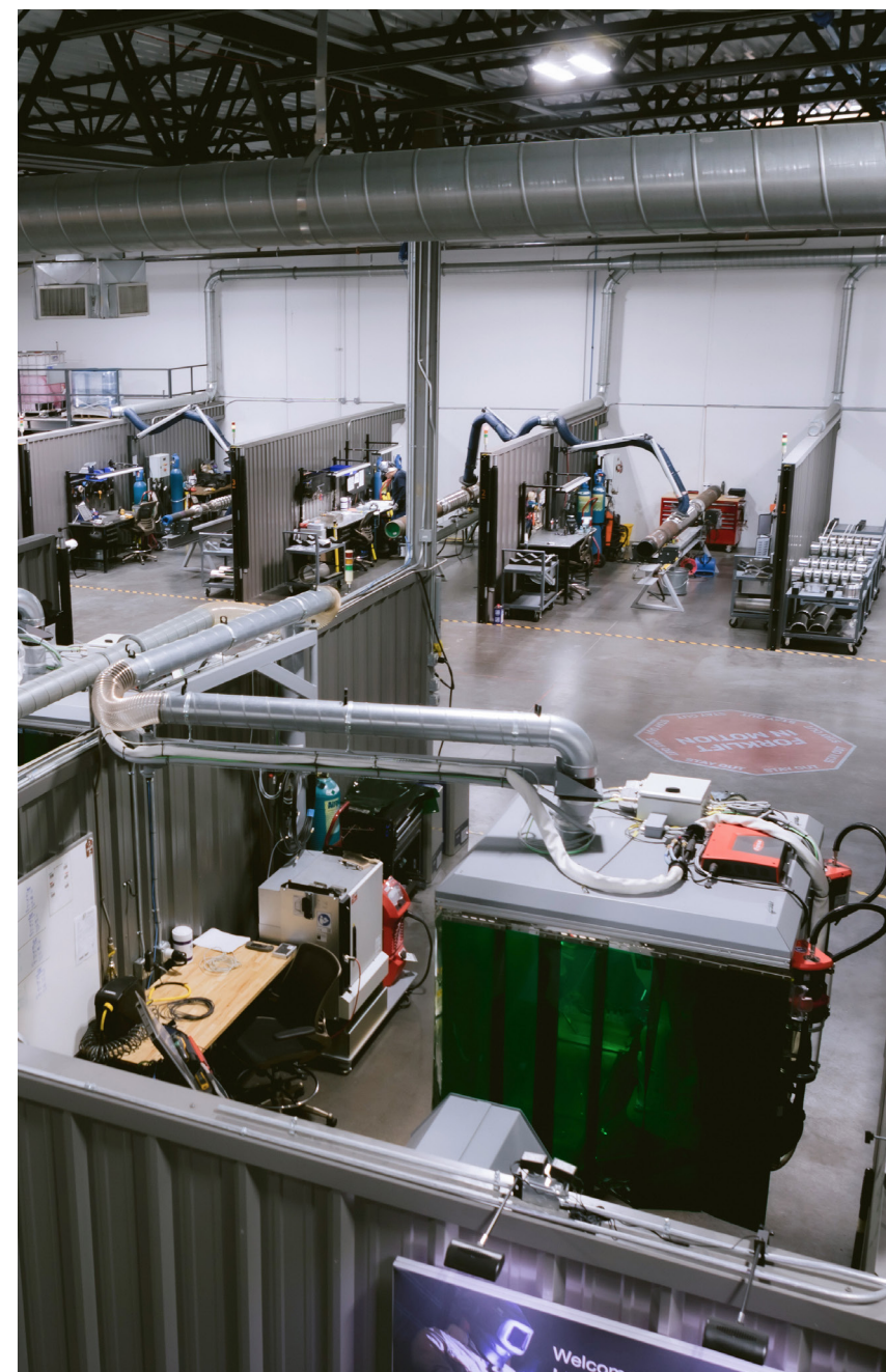
Newly established automated welding area for completions products in Houston IMC, USA.
