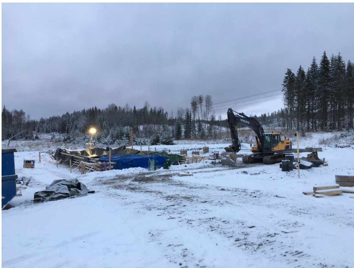
Etablering af transformerstation i Vindpark Knöstad (Sverige), 8 x SGRE 170 (6,2 MW) Construction of transformer station in Wind park Knöstad (Sweden), 8 x SGRE 170 (6.2 MW)
