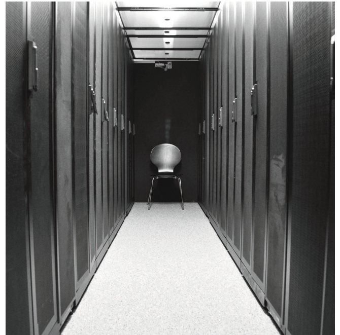
Sentia Denmark Services 2 A/S' Datacenter i Odense.
